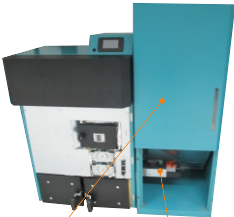
Position of pellet tank
